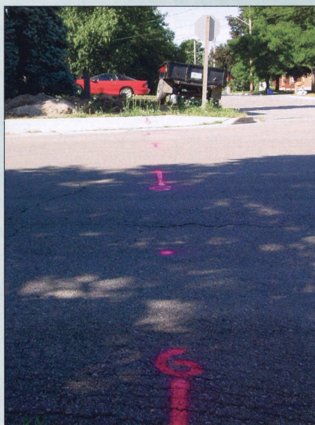
Figure 2: Annotated pink markings are used to mark Engineering Locates, or Level B SUE information. These markings show the inferred position of a gas main.
